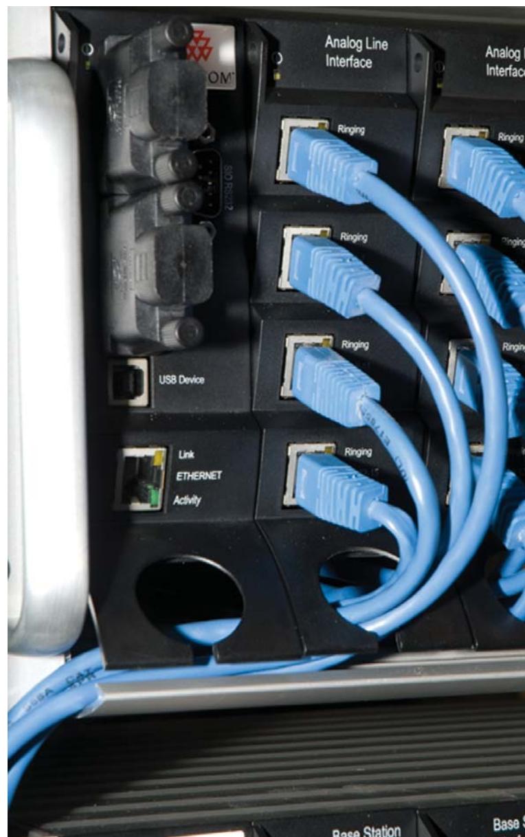
Figure 12 Harnessing cables to the side and out.
